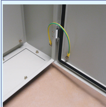
EARTHING BETWEEN BODY & DOOR
